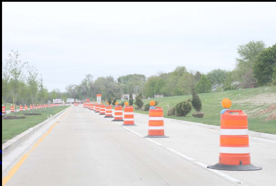
Crews continue to work on the Sandbloom Bridge and plant evergreen trees on LMP Section C-2 Sandbloom Rd to IL 25
