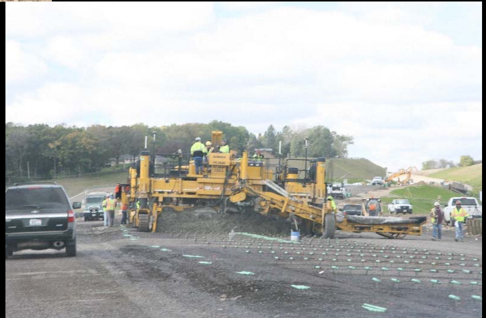
Crews pave portions of IL 31 in HMA and portions of LMP east of IL 31 in PCC on the LMP Section B-2 contract
