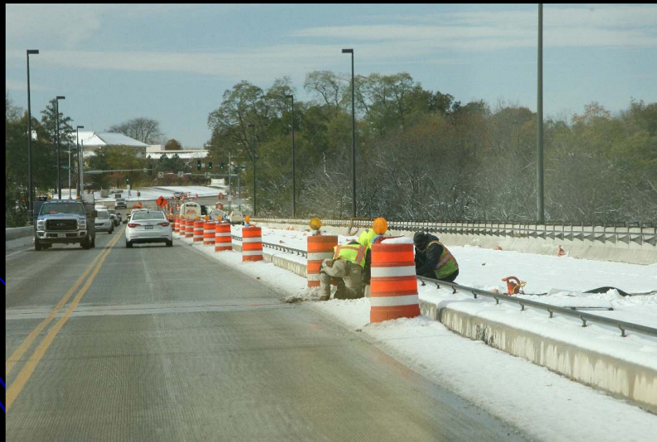
Crews prepare the bridge for the final deck pour on the Fabyan over Fox River Bridge improvement project
