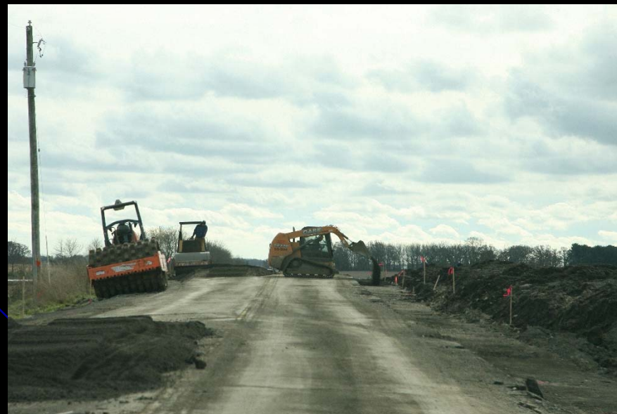
Crews continue shaping and grading the project site as part of the Peplow Rd over tributary to Virgil Ditch bridge replacement project
