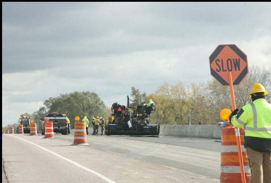
Crews pave the new ramp from Randall to US 20 as part of the Randall Road at Weld Road/US 20 intersection improvement project
