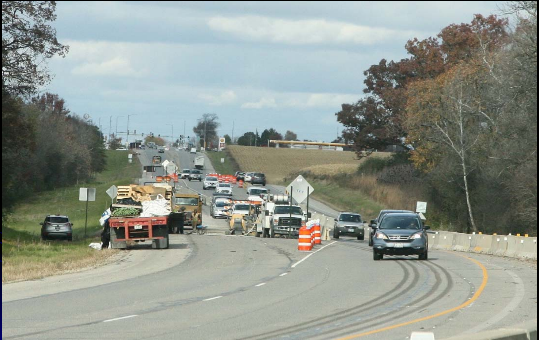
Crews remove the failed deck portion of the bridge on the Randall over Mill Creek Bridge Rehab project.
