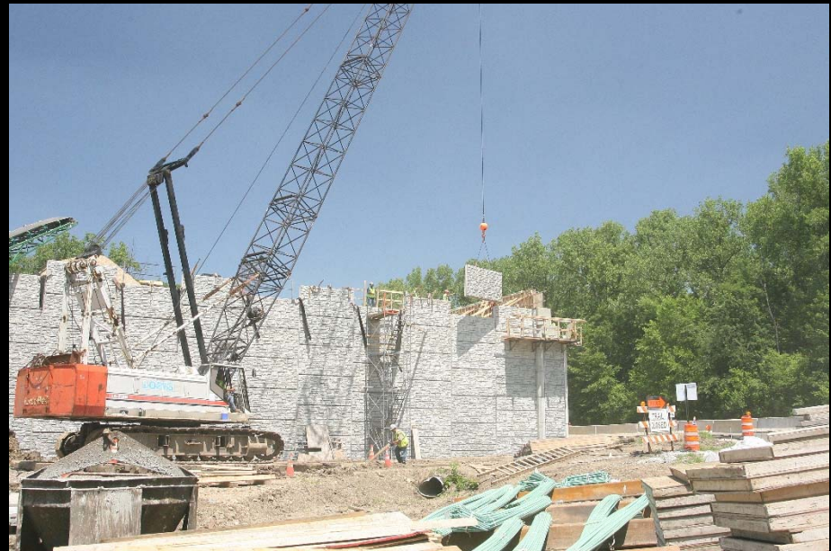
Crews continue building the east MSE island on the LMP C-1 new bridge over Fox River
