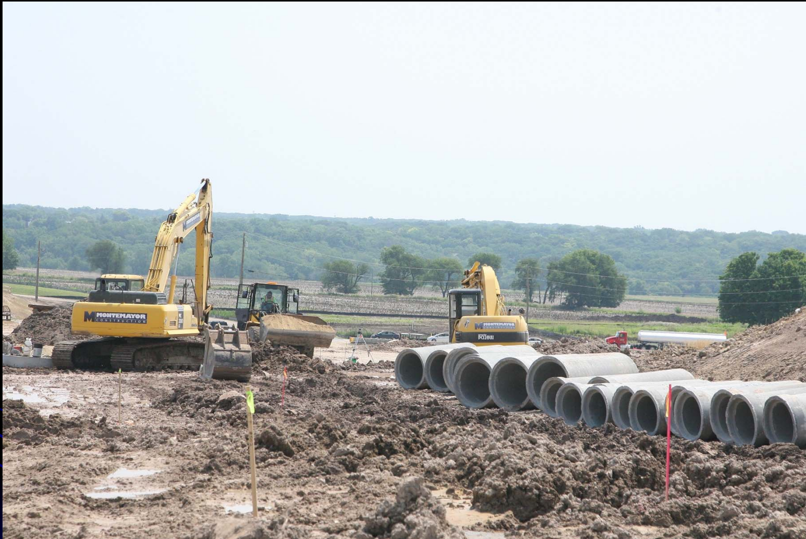
Installation of new storm sewer continues for the LMP Section B-2 contract
