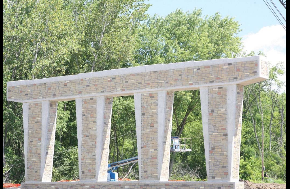
Crews continue form liner staining on the piers for the LMP C-1 new bridge over Fox River
