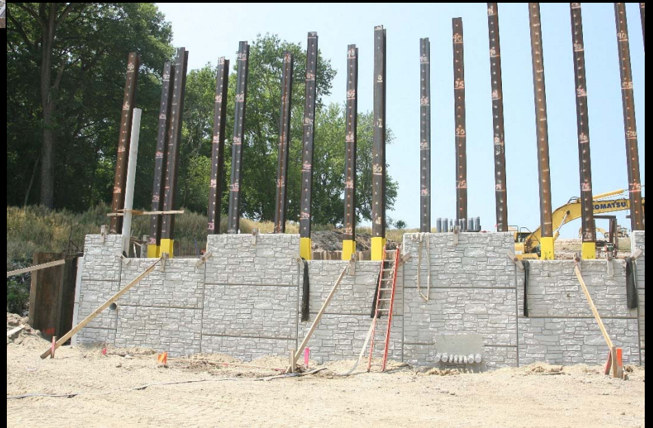
Crews work on the west MSE island for the LMP C-1 new bridge over Fox River
