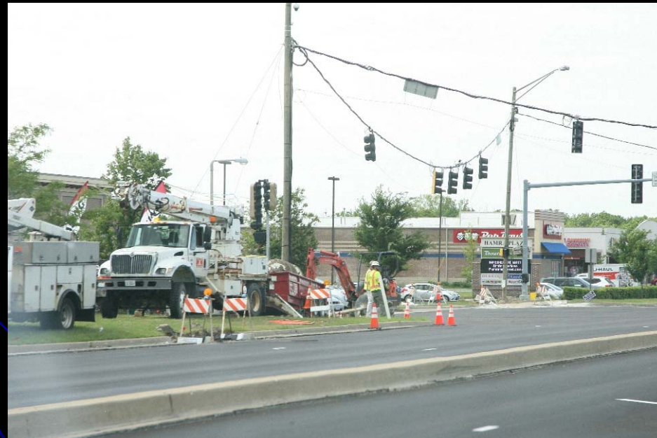
Crews instal new signals and ADA sidewalks at Kirk Rd at Mesa Rd as part of Kirk Rd – IL 56 to Cherry Ln Safety Improvement project
