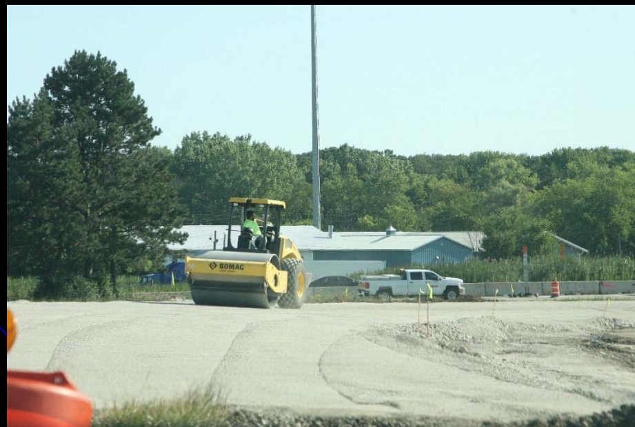
Crews install new storm sewer lines, pour wall foundation and work on constructing the new ramp to US 20 as part of the Randall Road at Weld Road/US 20 intersection improvement project
