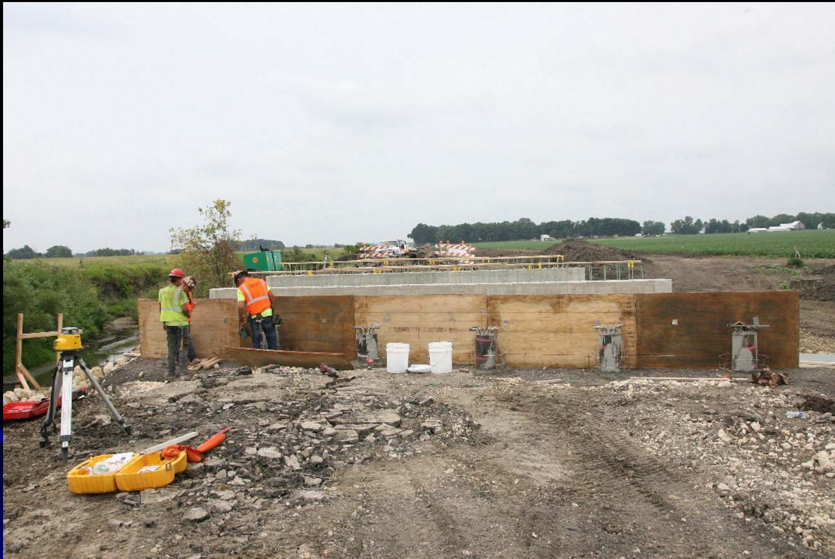
Crews begin constructing the substructure for the new bridge as part of the Peplow Rd over tributary to Virgil Ditch bridge replacement project
