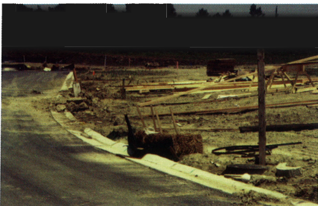
Construction site demonstrating the need for erosion/sediment control
